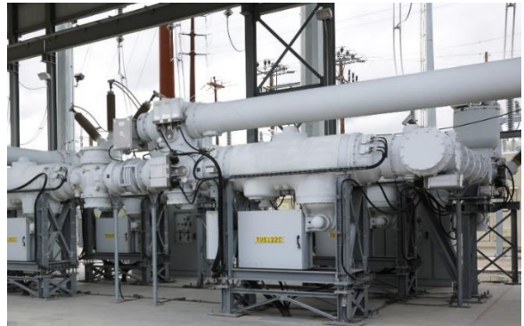
At TEP's Tucson Substation, circuit breakers and other electrical equipment are enclosed in conduit.
