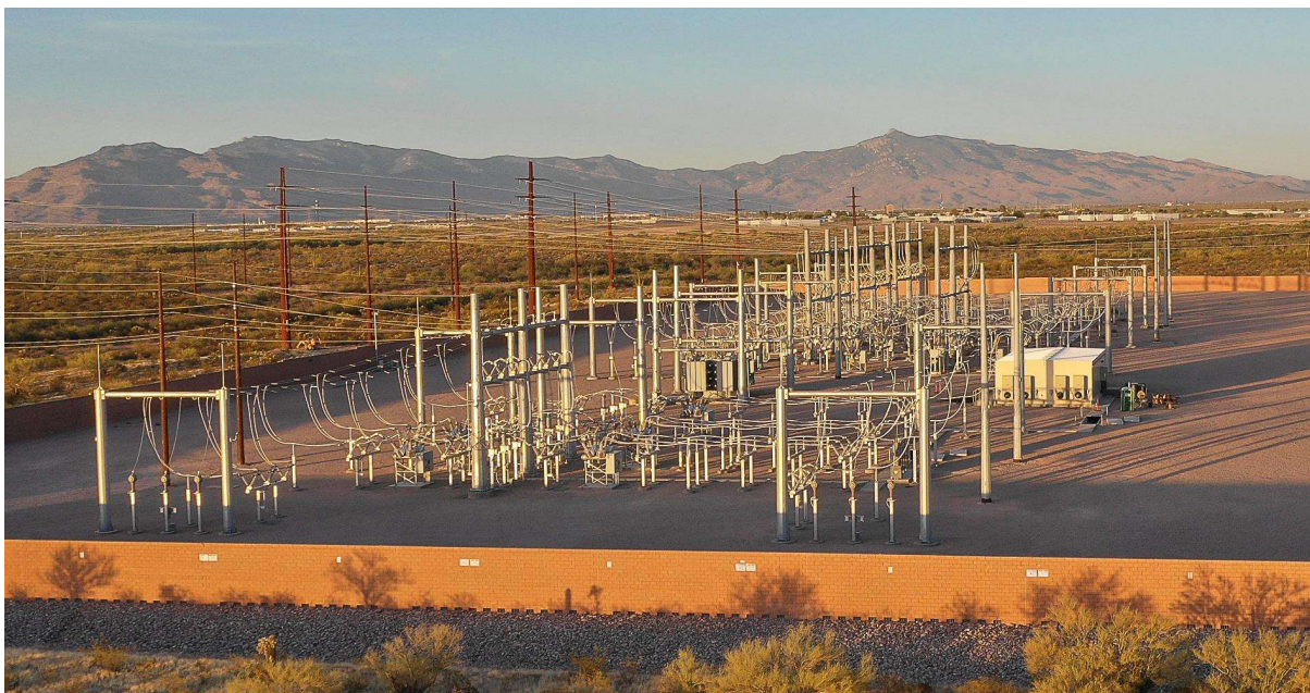
Existing Sonoran Substation
