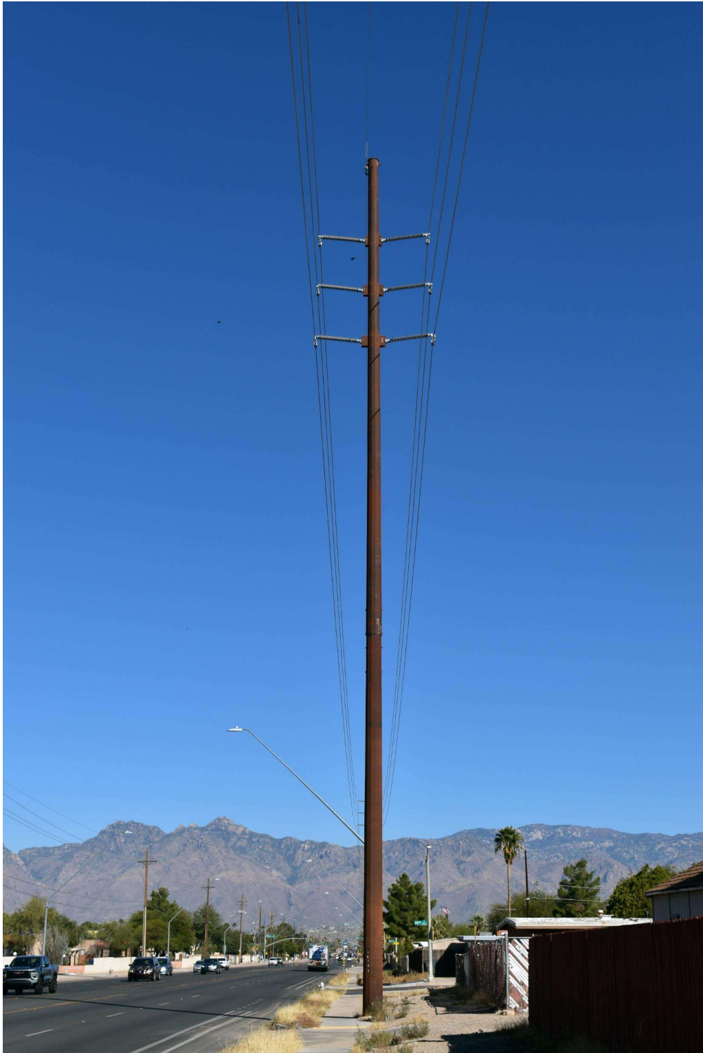
Typical structure, approximately 74 feet in height, located at 967 S Pantano Rd in Tucson.
