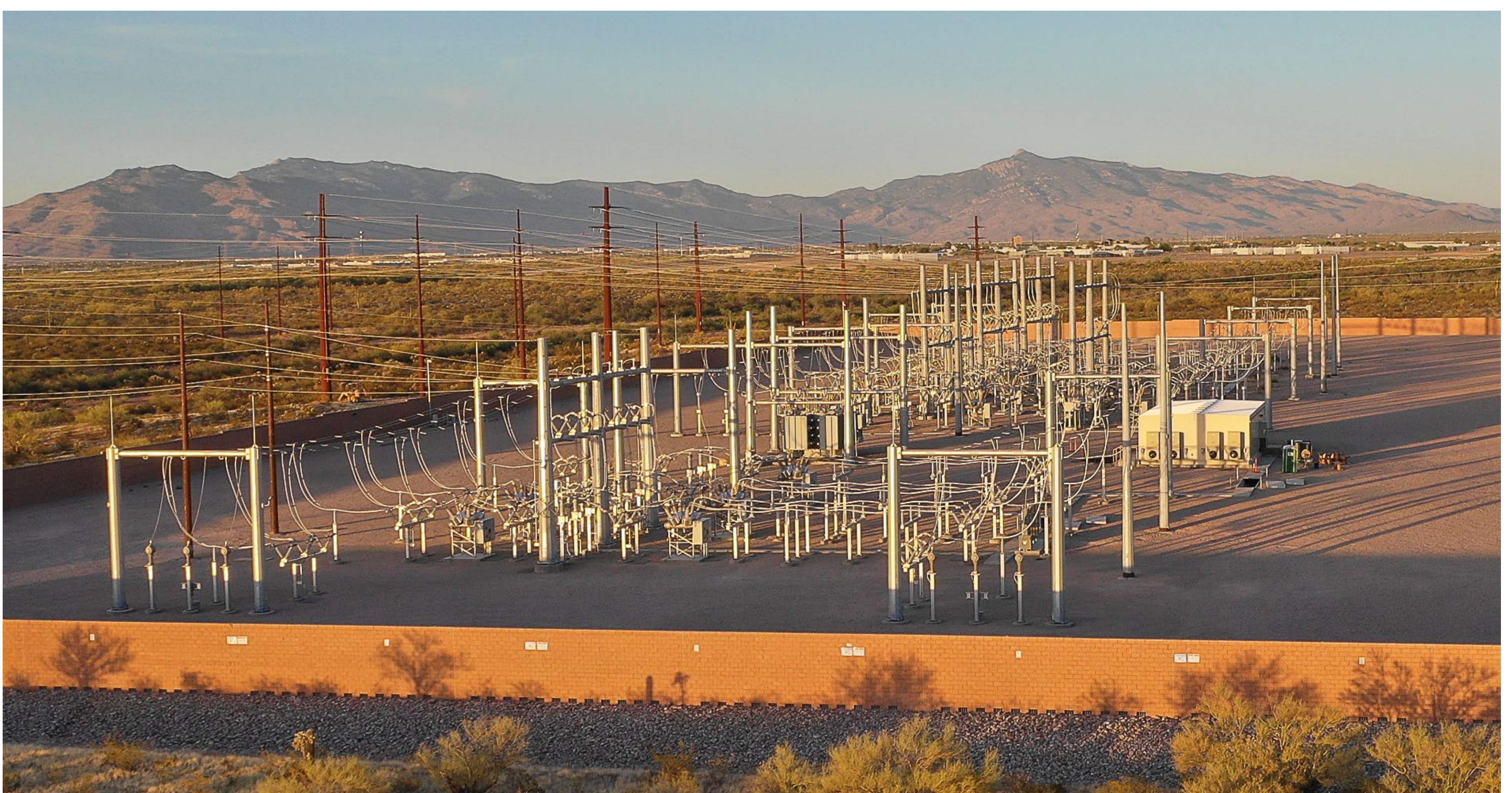
Existing Sonoran Substation
