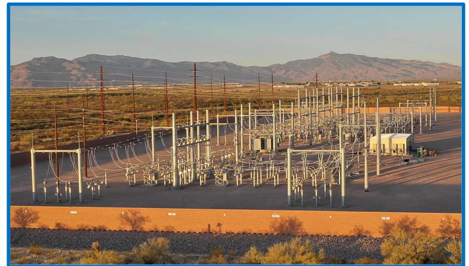
TEP's Existing Sonoran Substation
