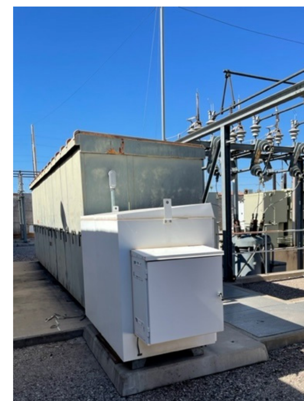
North Alvernon Control Shelter
