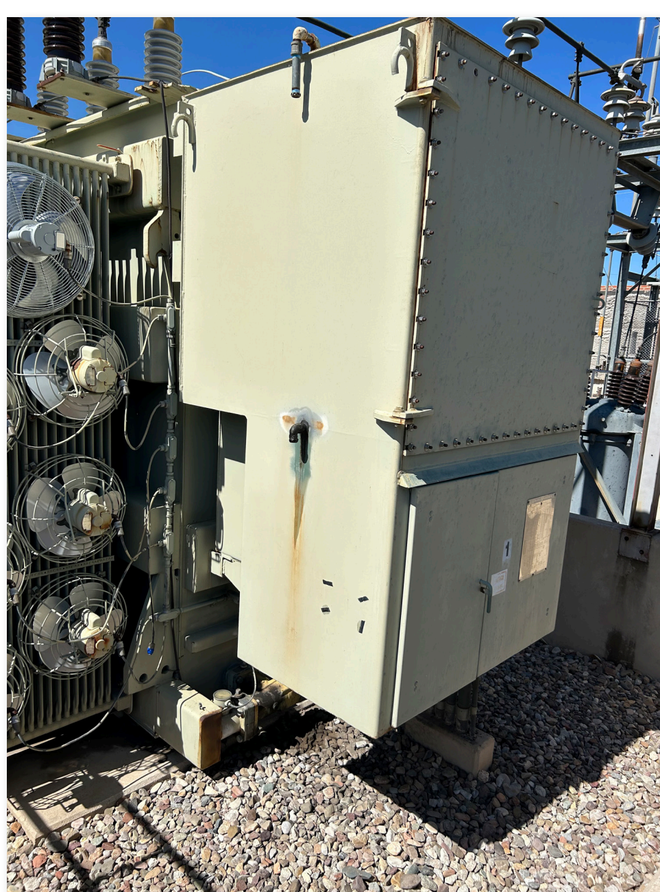
North Alvernon 46 kV to 4.2 kV Transformer
