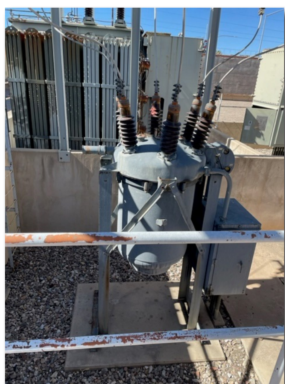
North Alvernon 46 kV Circuit Breaker
