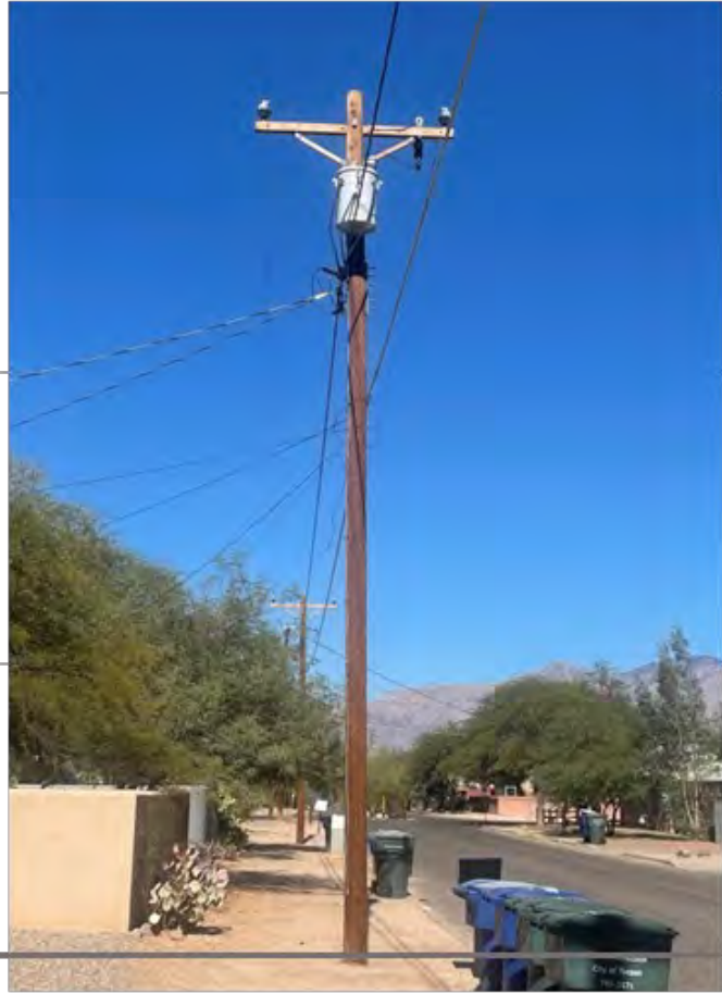
30' Distribution Pole (1300 N Camilla Blvd)
