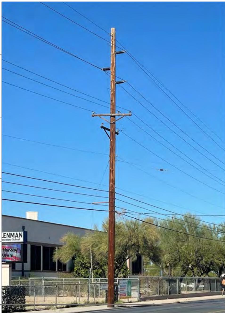
43' 46kV/Distribution Pole (1604 N Country Club Rd)
