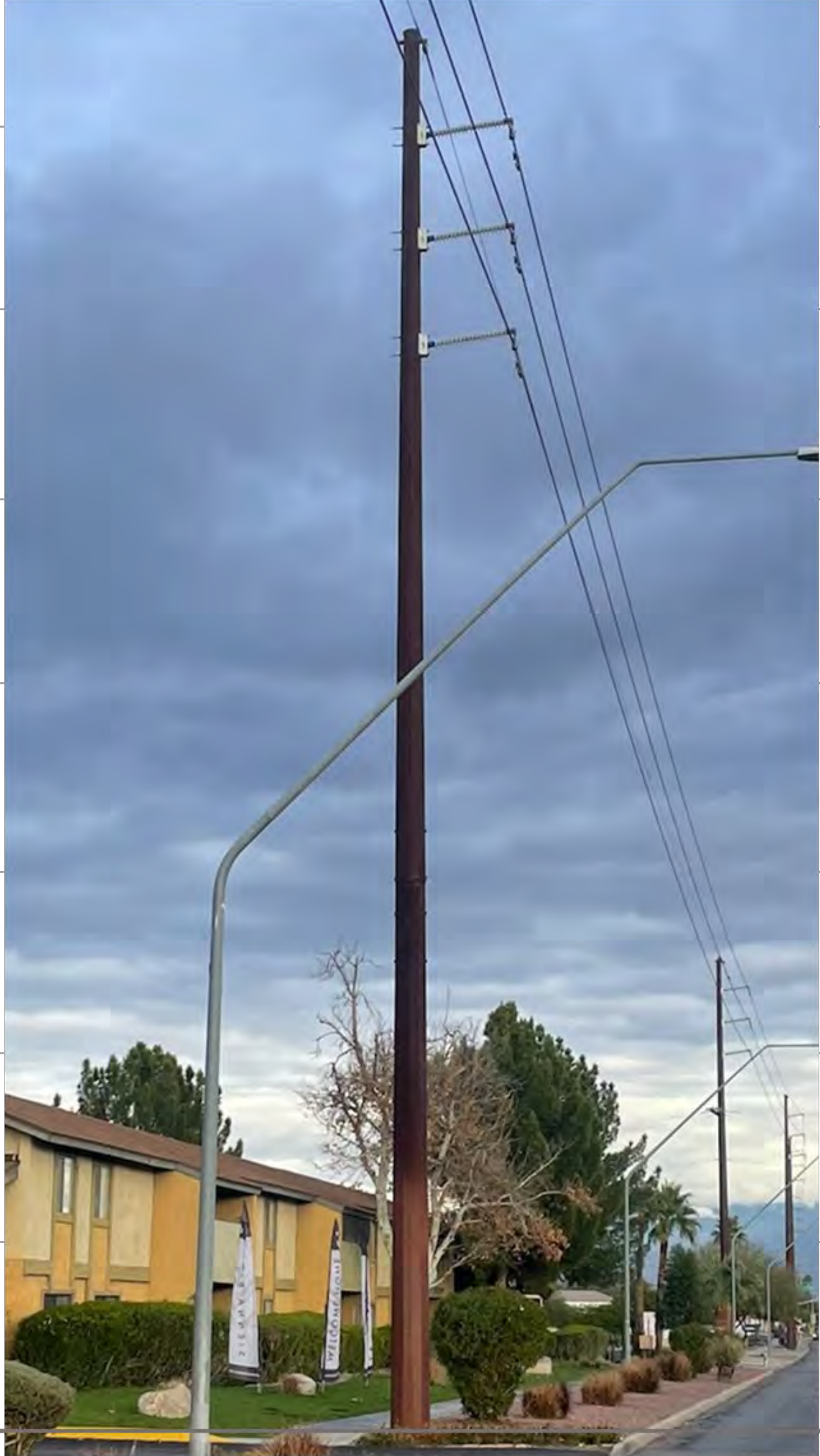
75' 138kV Transmission Pole (5353 E 22 nd St)
