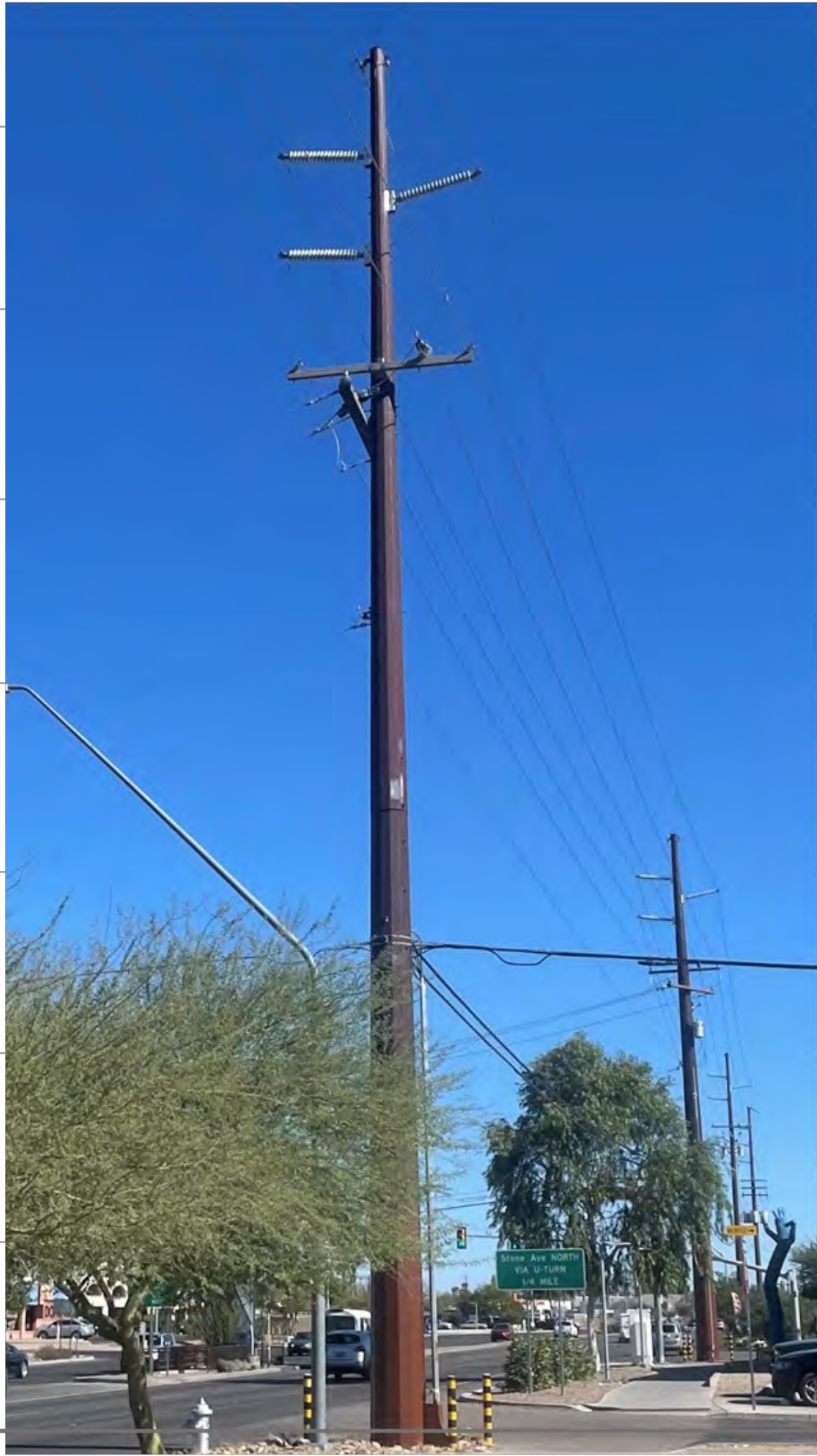
75' 46kV/Distribution Pole (201 W Grant Rd)
