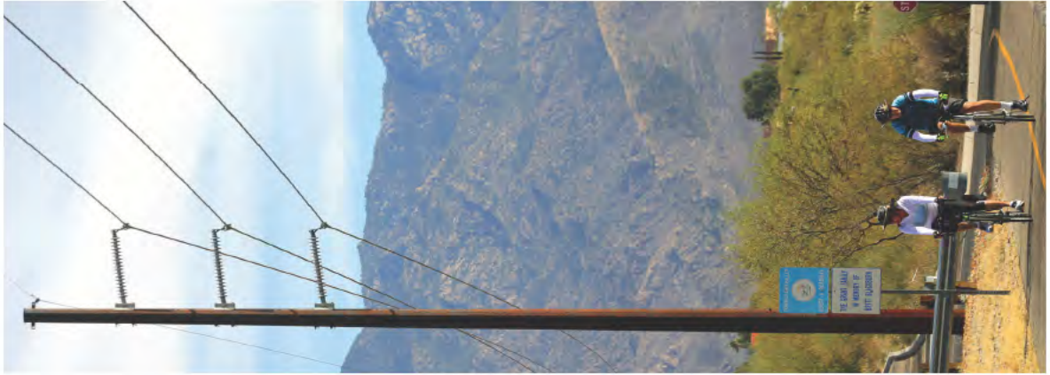
A typical weathering steel monopole supporting a 138 kilovolt transmission line
