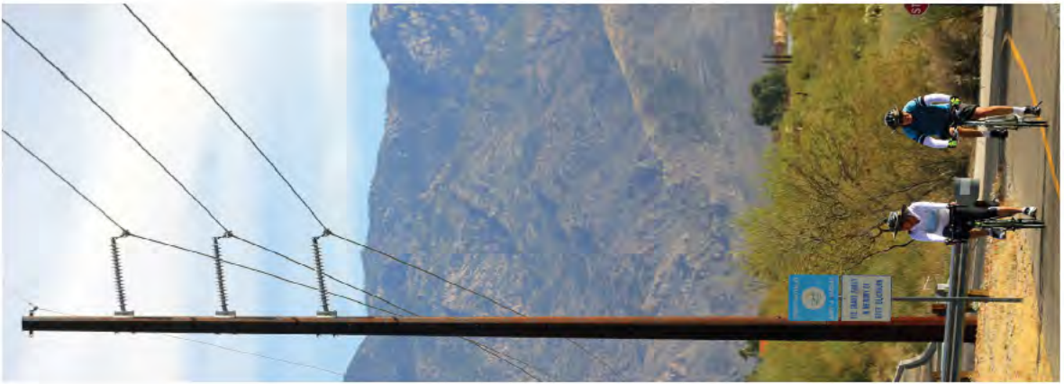
A typical weathering steel monopole supporting a 138 kilovolt transmission line
