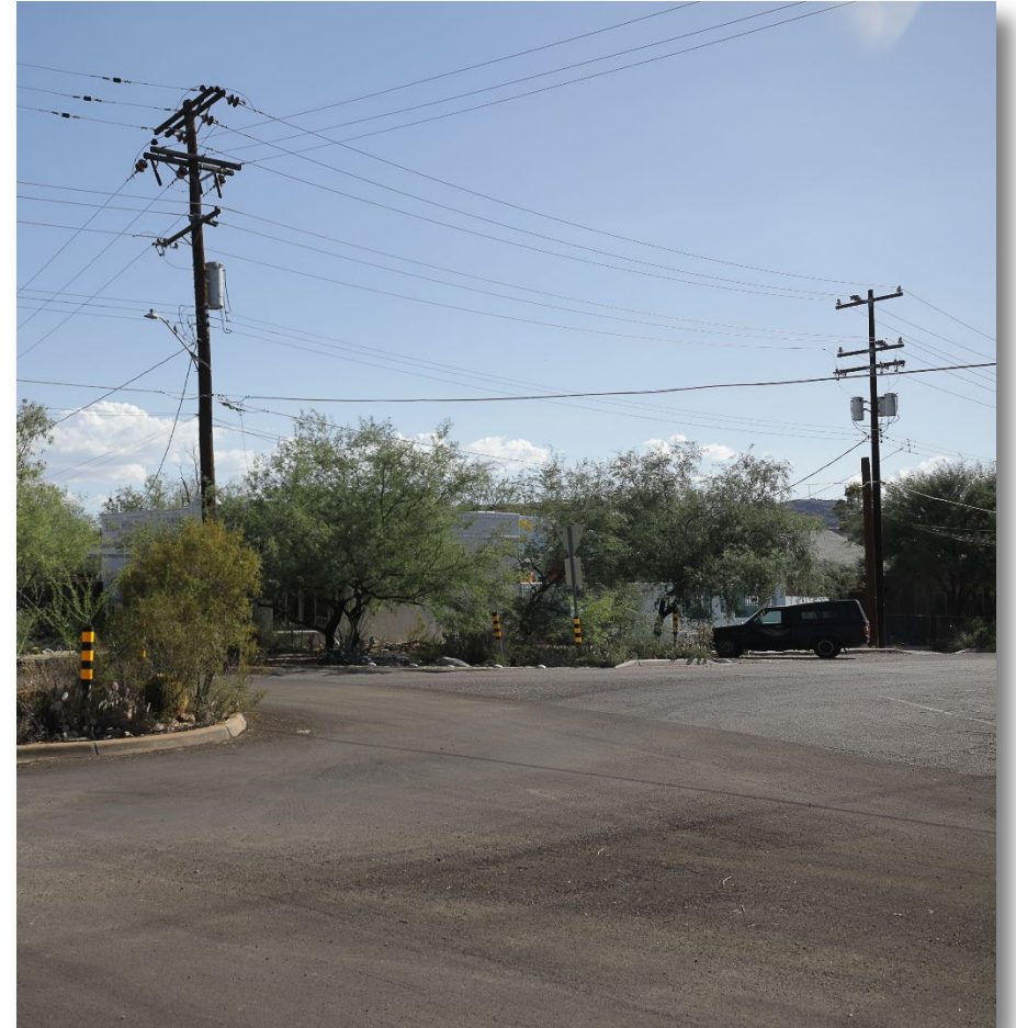
Existing 4kV distribution infrastructure at 4 th St. and 9 th Ave.
