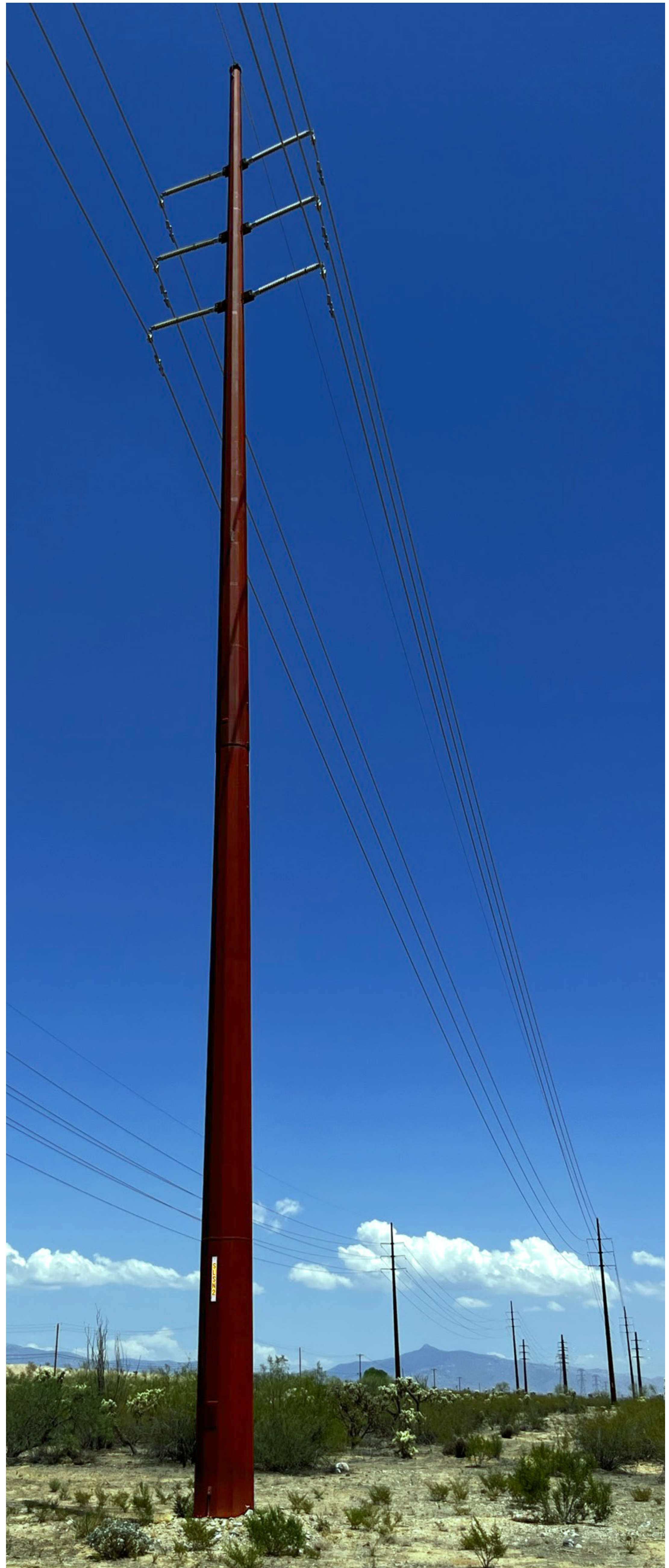
A typical weathering steel monopole supporting a 138 kilovolt transmission line
