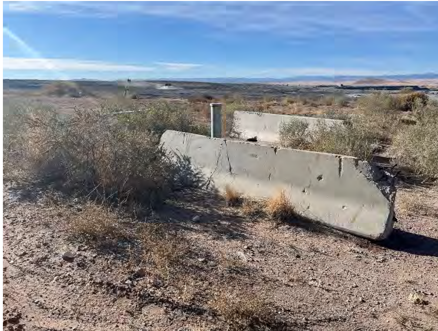
Photo 3 Condition of Groundwater Monitoring Well, CCR-2U; facing southwest
