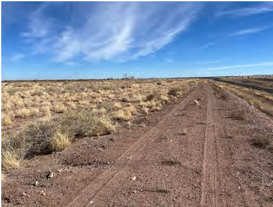
Photo 36 Typical conditions along outer edge of the top bench of the landfill; facing east
