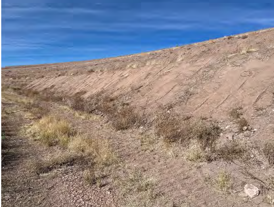
Photo 47 Repaired erosion rills on side slope of Inactive Fill Area; facing northwest
