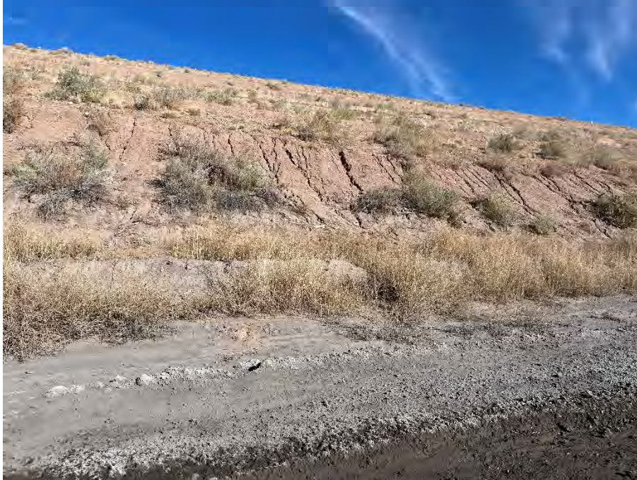
Photo 35 Erosion rills along south slope near the Ash Haul Road; facing north
