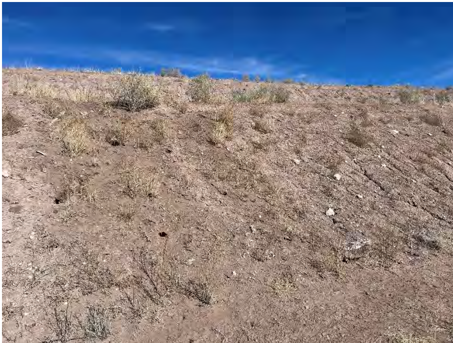
Photo 24 Animal burrows and minor erosion rills present on side slope; facing north
