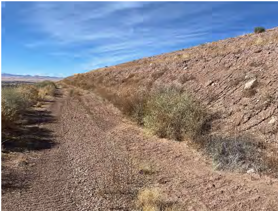
Photo 52 Erosion rills on the slope; facing west
