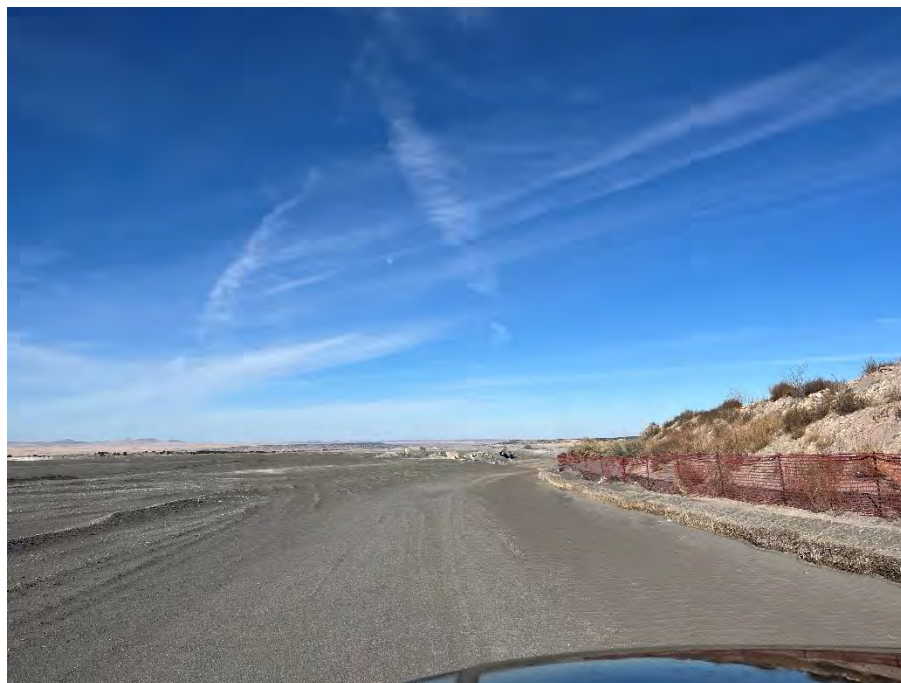
Photo 4 Typical conditions of perimeter access road and erosion and sediment controls (e.g., orange construction fence and hay bales) to northwest portion of landfill; facing northwest
