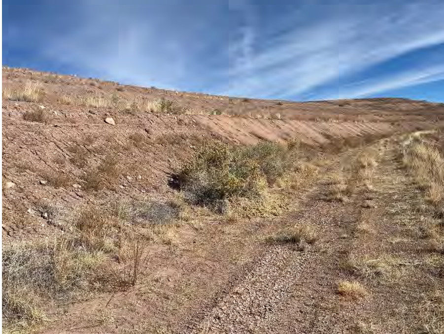
Photo 49 Typical conditions and repaired erosion on side slope; facing east
