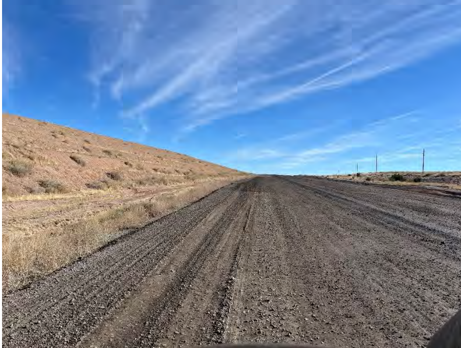
Photo 21 Typical condition of Ash Haul Road; facing east
