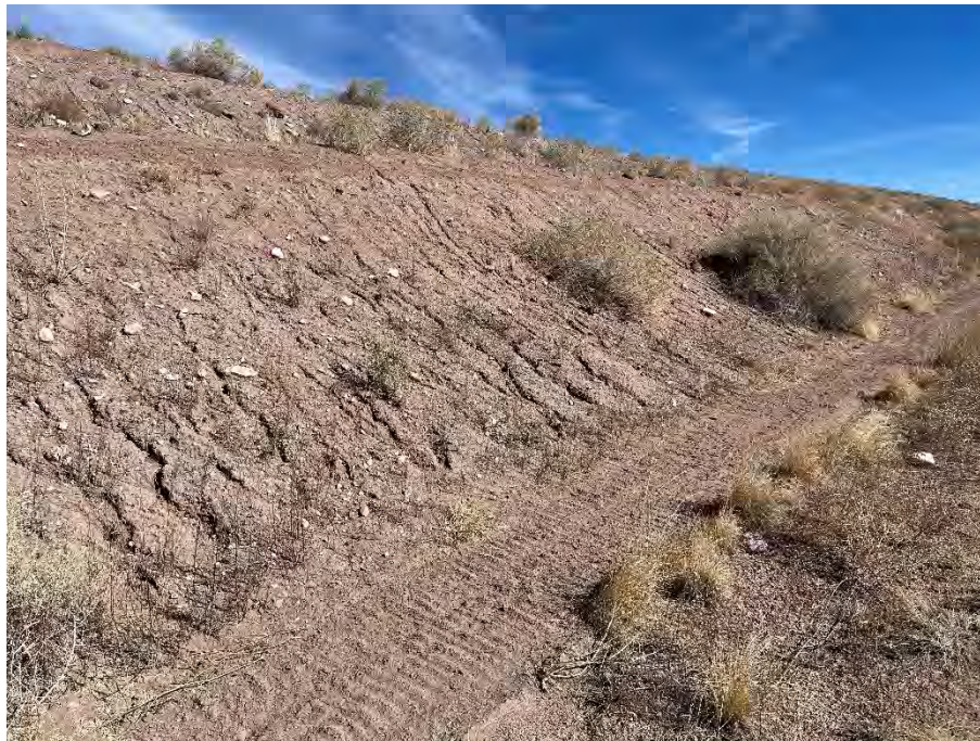
Photo 40 Erosion rills on side slopes; facing northeast
