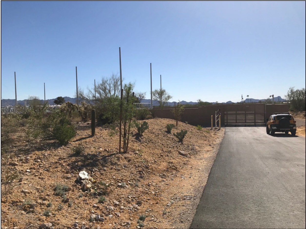
Photo 1. Orange Grove Substation at Orange Grove Rd. and La Cañada Dr., looking west.
