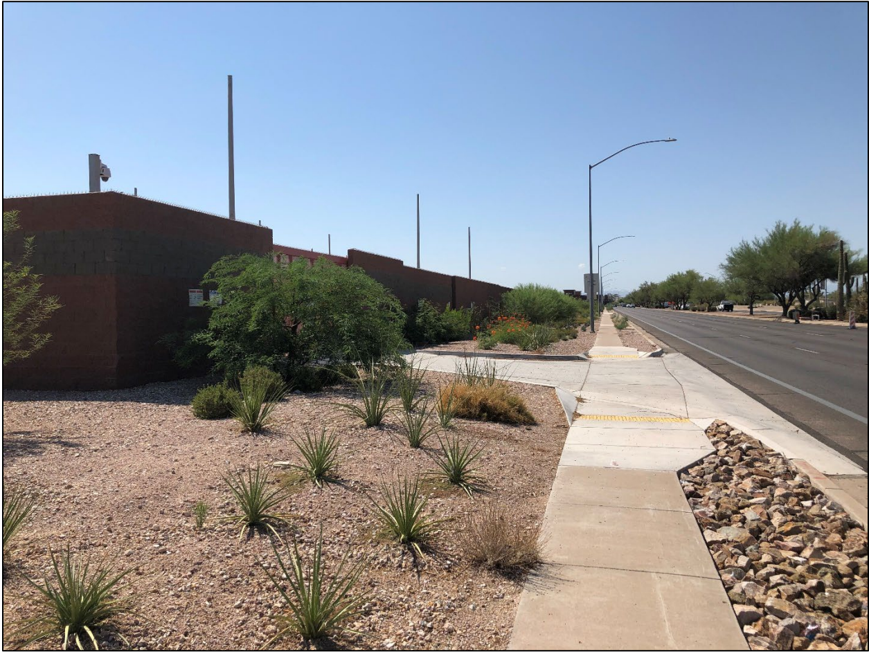
Photo 2. Kino Substation at 36th Street and Campbell Ave., looking south.
