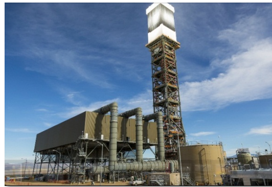
Ivanpah Solar Receiver and Condensers
