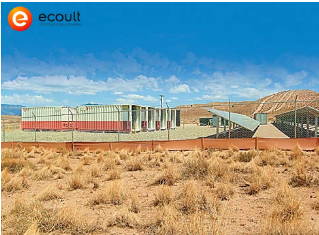
Picture 14 – PNM Prosperity Energy Storage Project
