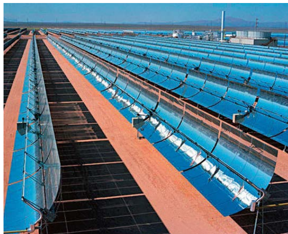
Harper Lake Solar CSP Project (NREL)
