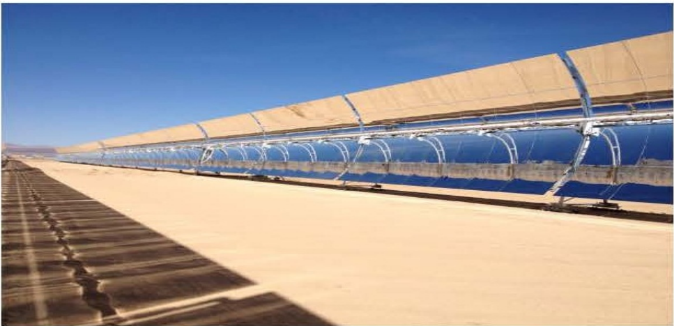
Mohave Solar Collectors
