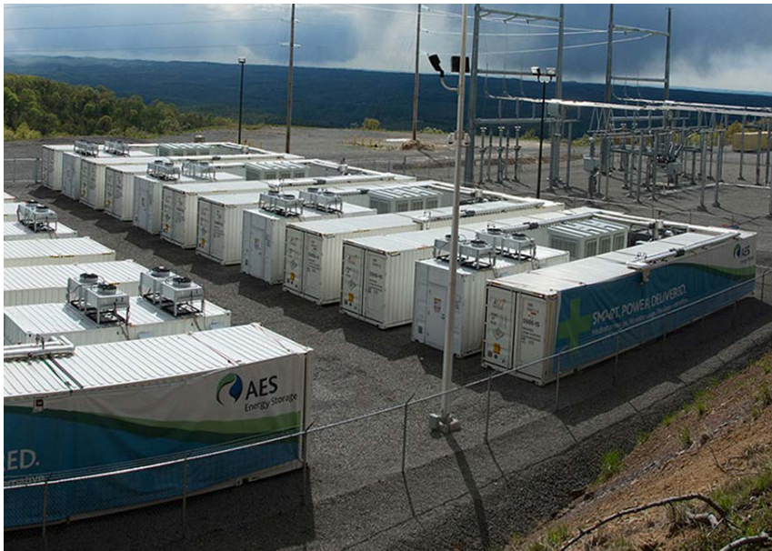
Picture 17 - AES Storage LLC's Laurel Mountain Energy Storage Supplies 32 MW of regulation using Li-ion batteries
