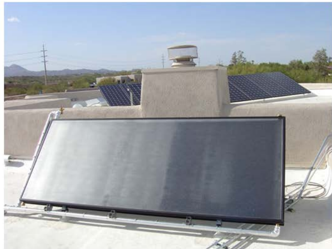
Typical solar hot water heater system
