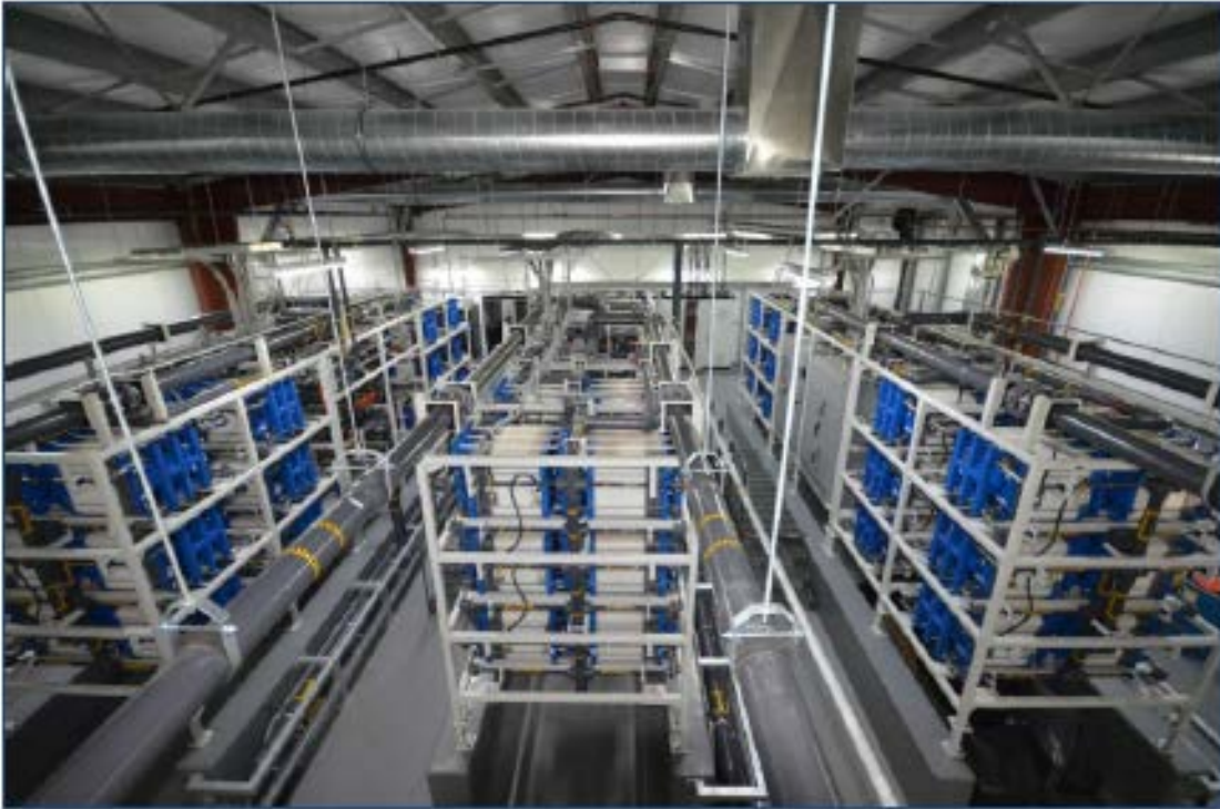
Picture 18 – Prudent Energy Vanadium Redox Flow Battery Project
