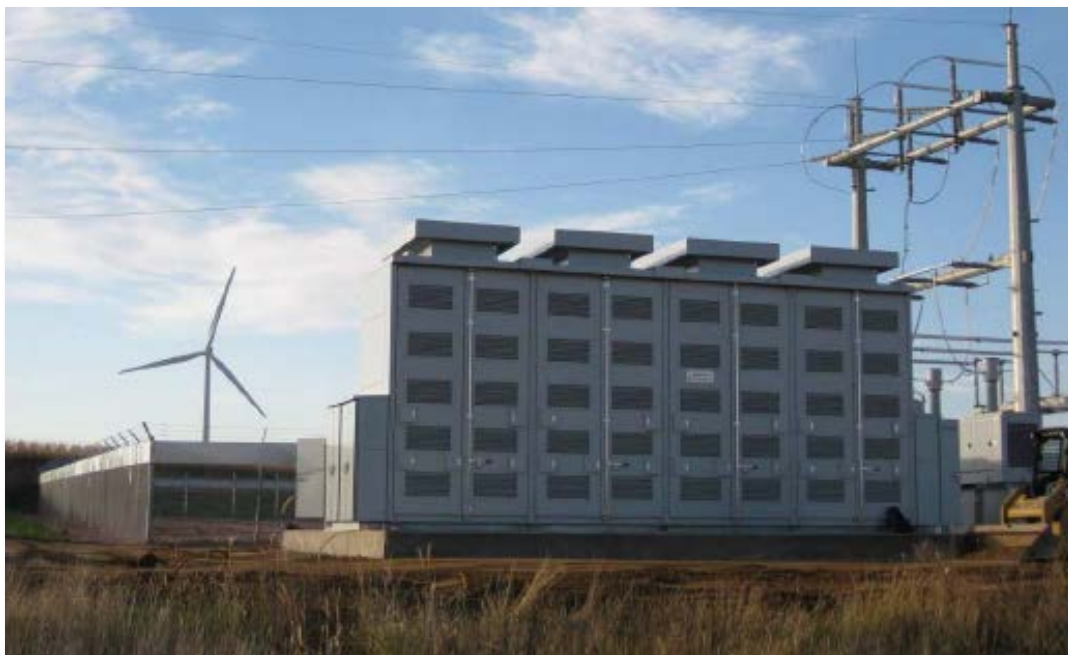
Picture 16 - Xcel Energy – Wind to Battery Project
